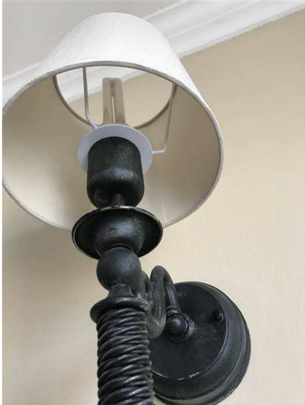
Various lighting in hotel: CFL
