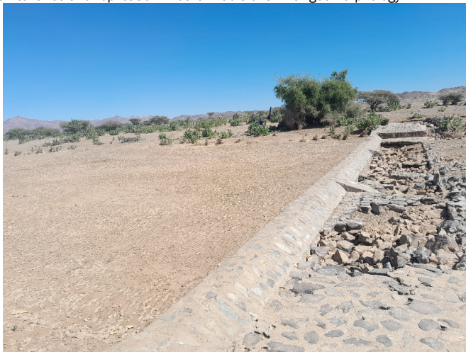
Figure 4 Anikwan dam in 2025. While the dam main body is in good condition, downstream energy dissipator requires urgent maintenance.
