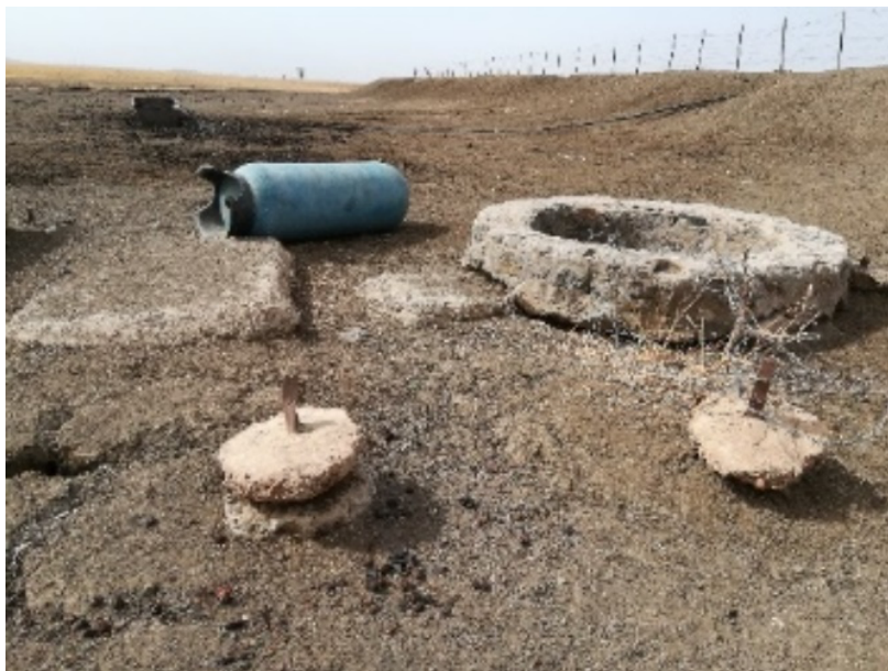
Figure 6 Broken outlet well and treatment unit of a Hafir in Al-gadarif. Source: field work
