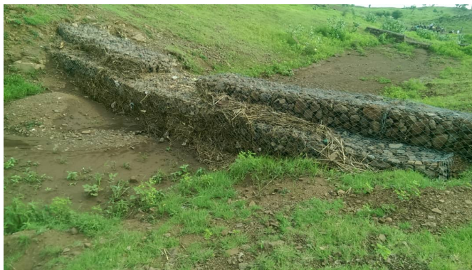
Figure 42 Umsenibra check dam
