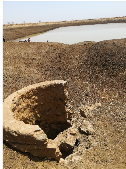
Figure 8 Damage inlet system in A Hafir, Al-Gadarif. source: Field work
