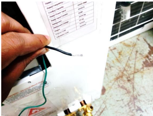
Before: Soldered wire terminal strands
