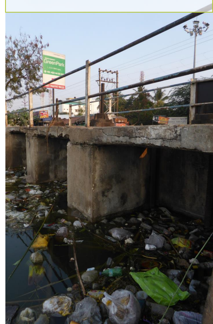
Poor lake infrastructure
