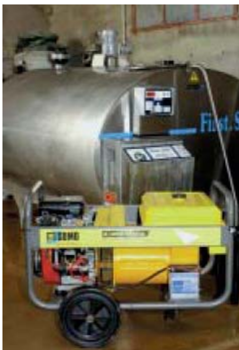
Figure IP06/5. Portable Diesel Generator
