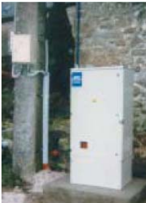
Figure IP06/1. Voltage regulator
