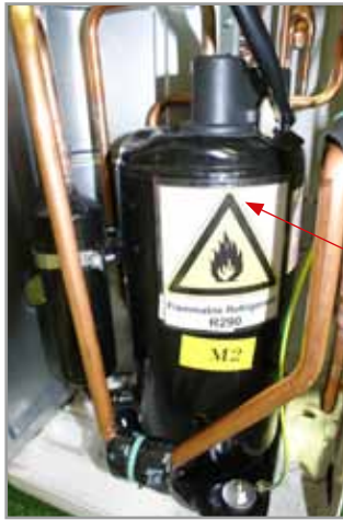
Figure 30: Warning sign at the compressor
