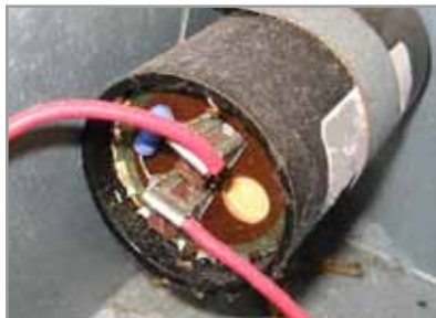
Figure 23: Not acceptable capacitor may cause short-cut and sparks
