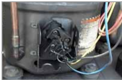
Figure 22: Loose connection causes arcing and short-cut
