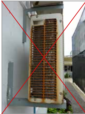
Figure 10: Example of AC system that is unsuitable for conversion
