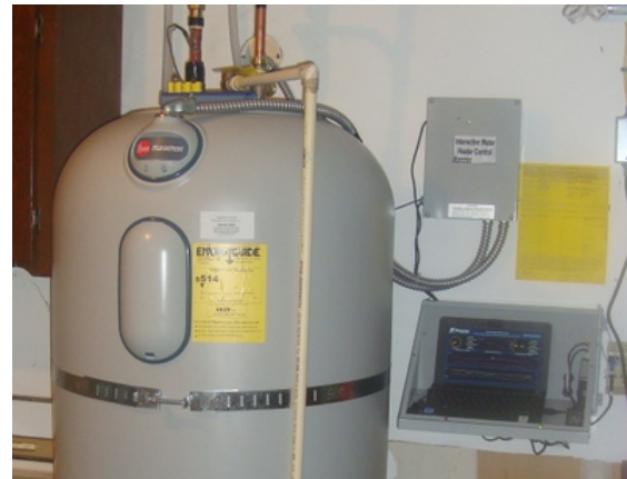
Figure 5: Installed 105 gallon water heater with Steffes™ mixing valve and interactive controls
