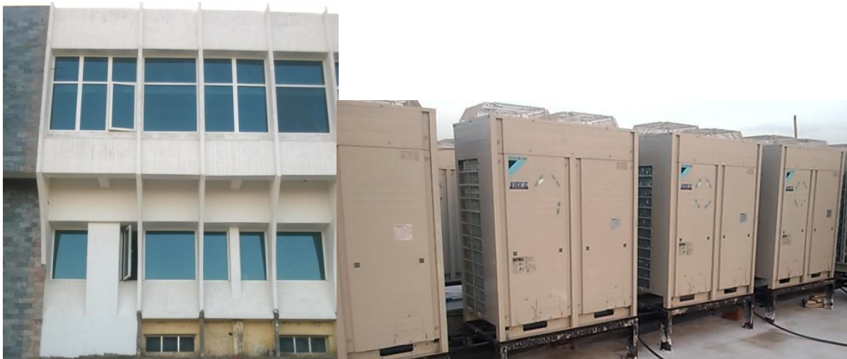
Figure 26 : 3 Pane windows (Left) and VRF Air Conditioner Units (Right)
