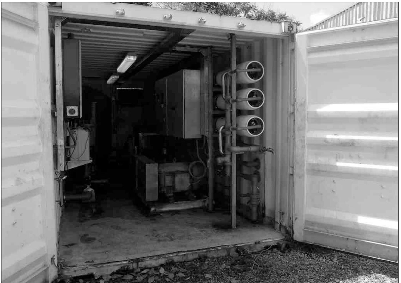
One of three containerised RO units near the Nauru power station. Source - SOPAC 2009
