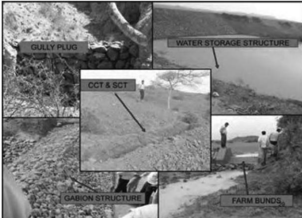
Rain Water Harvesting Structures
