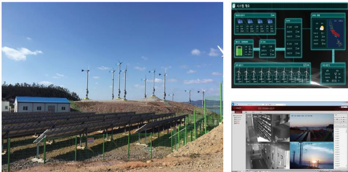
Figure 2. Samma Island Hybrid Renewable Microgrid System (PV + Wind + ESS)
