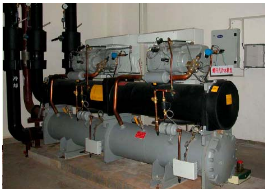
Fig.5 Multi-stages AC chillers
