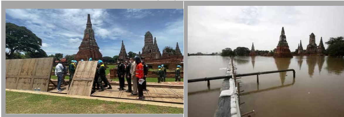
Movable flood gates being erected during pre-flood conditions and during flood situation.
