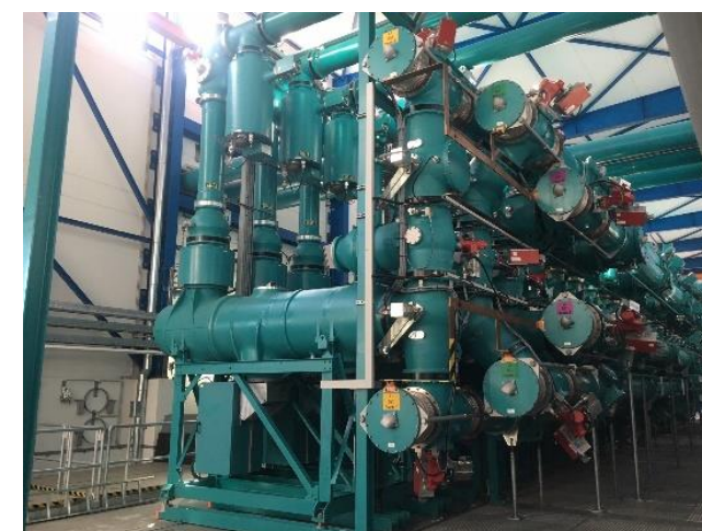
Gas insulated switchgear (GIS)
