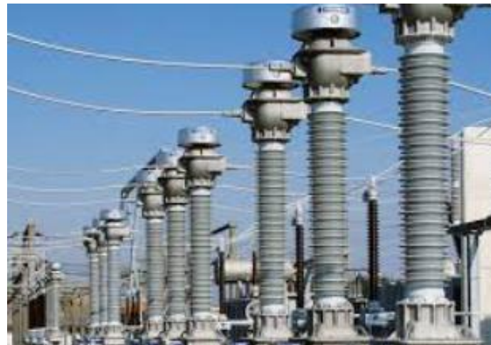
Instrument transformers (IT)
