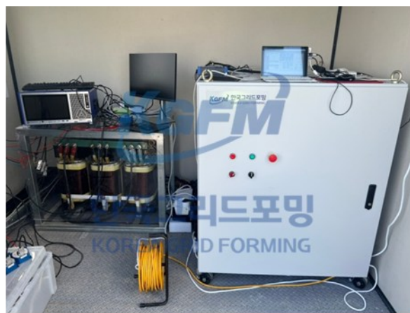
Installed GFM inverter
