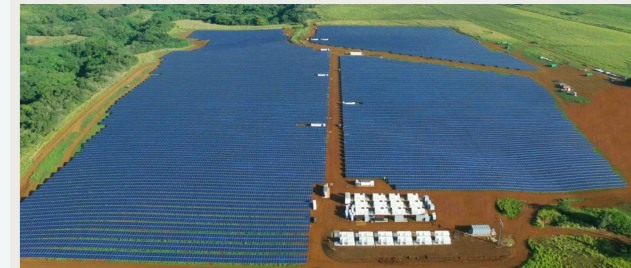
The photovoltaic panels at the Kapaia solar-plus-storage facility, operated by the Kauai Island Utility Cooperative in Hawaii, are capable of generating 13 megawatts under ideal conditions. TESLA
