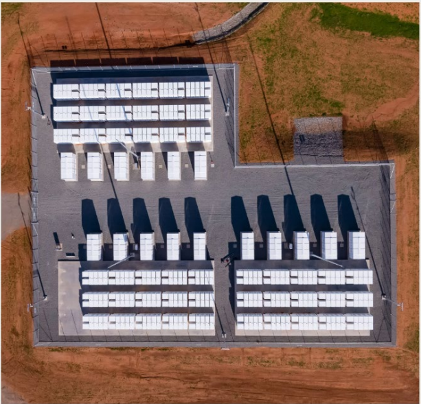
Hornsedale Power Reserve, Australia — 150 MW / 194 MWh, grid-forming
