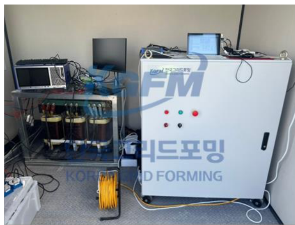
Installed GFM inverter
