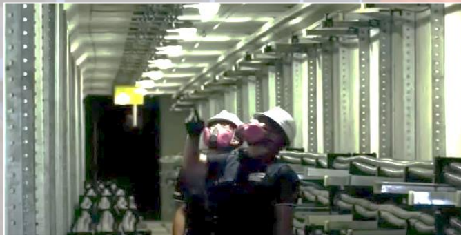
Worker's underground power grid inspection site
