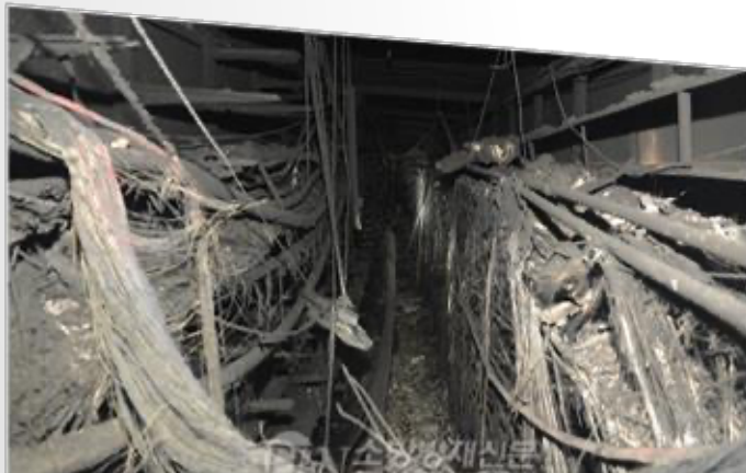
KT Ahyeon Branch Communication District Fire
