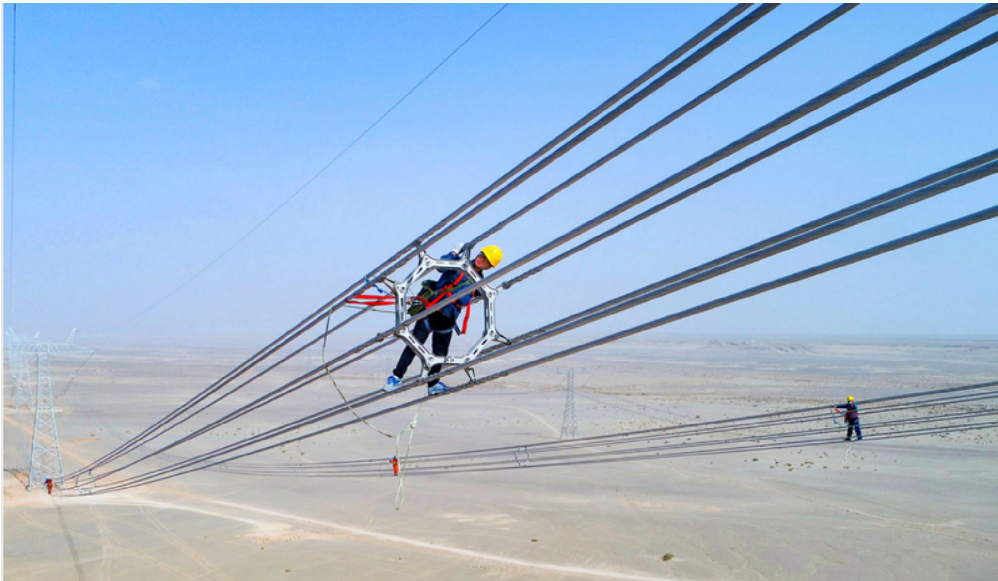
Crushing It: China's newest UHV line from Xinjiang to Anhui has set world records for transmission distance, power, and voltage. PHOTO: VCG/GETTY IMAGES
