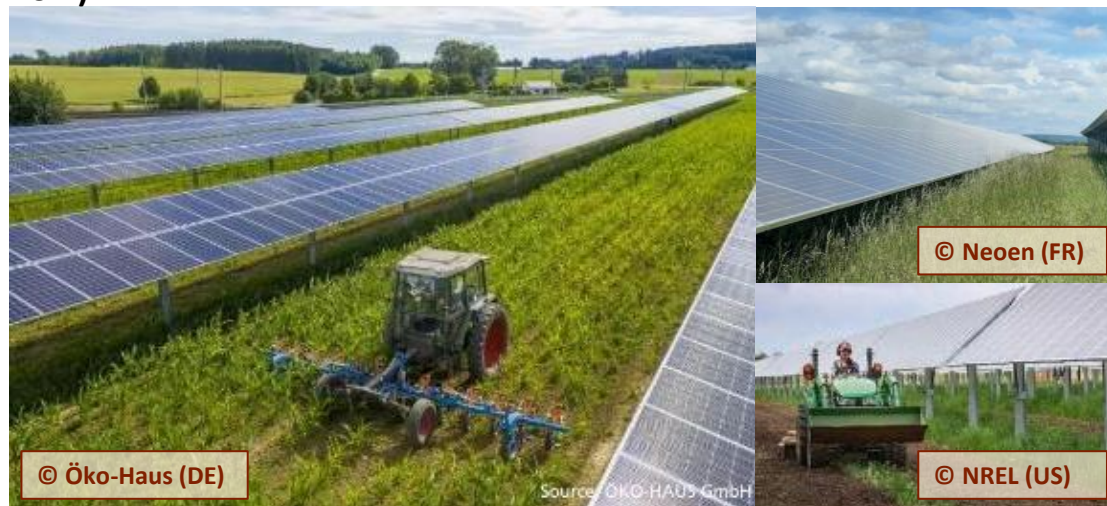
Ground-mounted PV systems with crops between rows of modules (inter-row)
