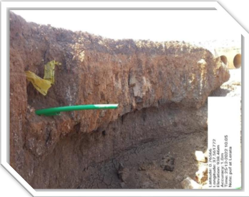
Flashfloods sever fiber optic cables in the Philippines, 2022
