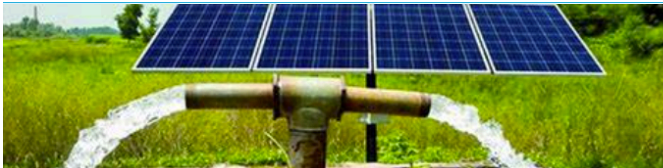
Example of Solar Powered Irrigation System with pump. © UNEP-CTCN
