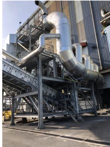
Ash re-introduction into boiler (system not working at the time of site visit)
