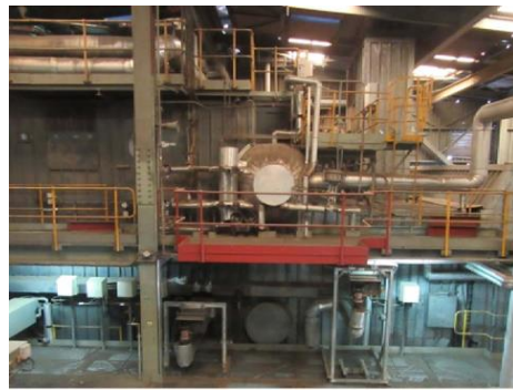
Boiler Steam and Mud Drums & Steam headers
