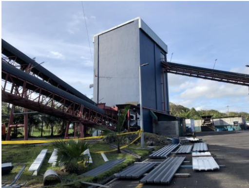
Coal handling conveyors
