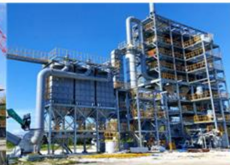
Installation of environmental pollution prevention facilities
