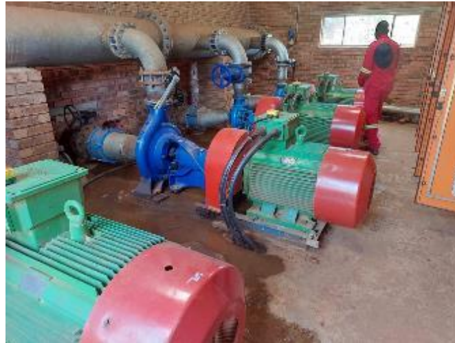
Figure 8 - Pumps of Mnyangombili Farm
