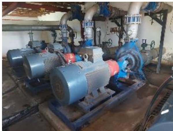
Figure 16 – Pumps of Lomdashi Farms
