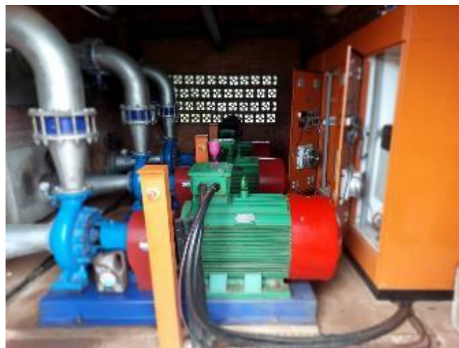
Figure 7 - Pumps of Mnyangombili Farm
