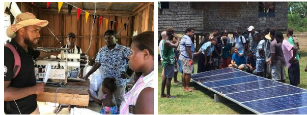
Figure 4: Moerk Water solar powered water treatment system installed at a Maternity clinic in Western Province in 2017 for drinking water. 4
