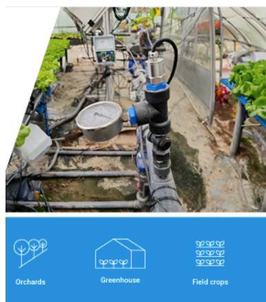
Figure 10. Pressure sensor installed in a greenhouse (Netafim, 2023).
