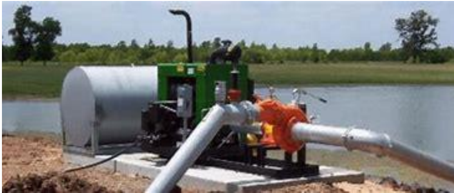
Pumping station on a river
