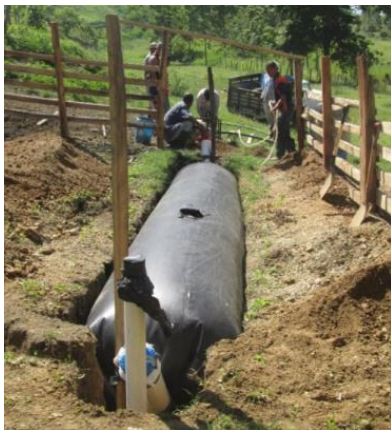
Figure 9. Tubular flexible roof biogas.
