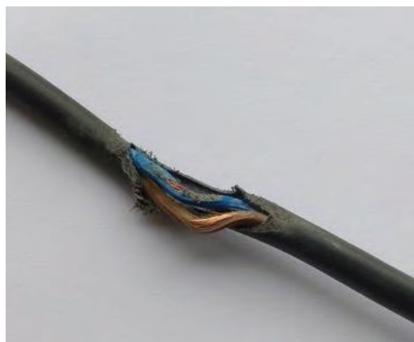
Figure 3: Damaged Insulation Requiring Immediate Replacement
