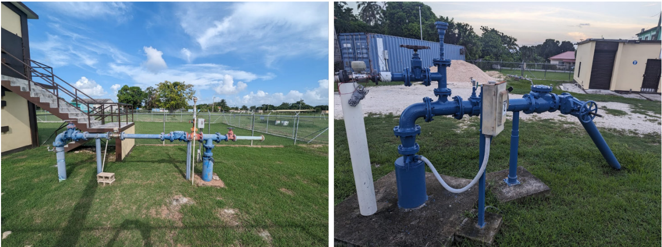
Figure 2.5: Example of Rural Water Supply (RWS) boreholes
