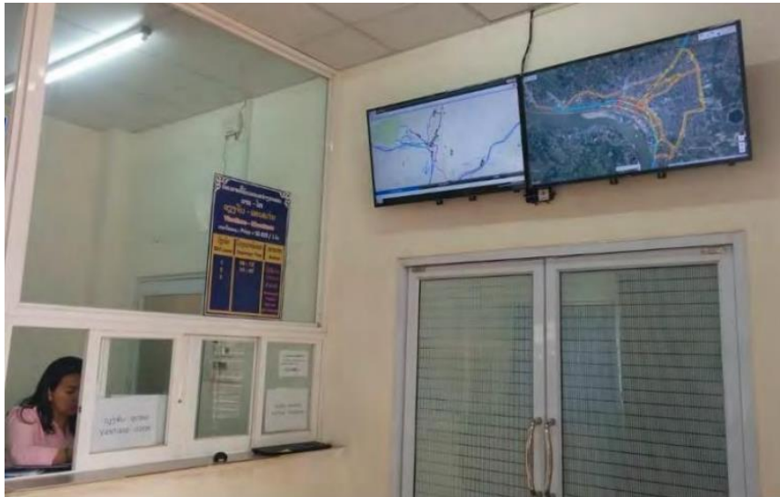
Figure 17: Customer-Facing Monitors at the CBS
