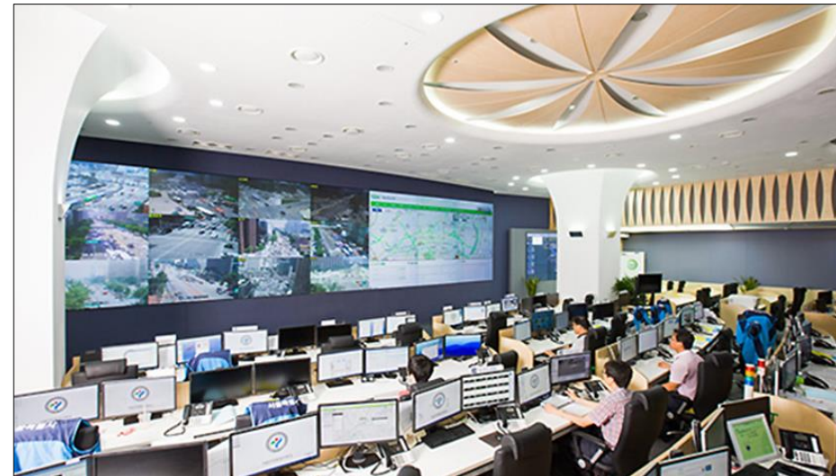
HQ monitoring centre (TOPIS)
