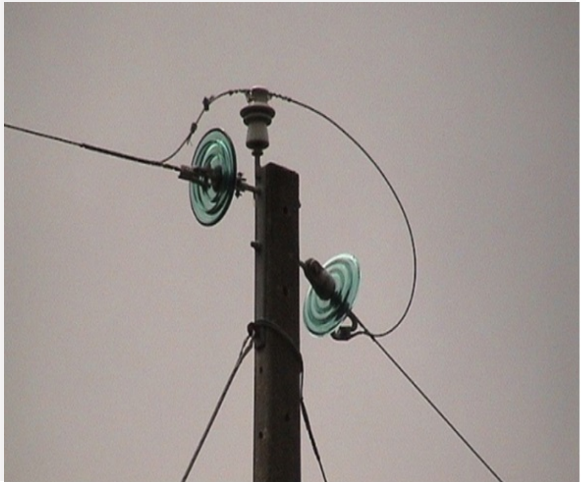
Figure 7: SWER pilot project (Source: REF, 2015)
