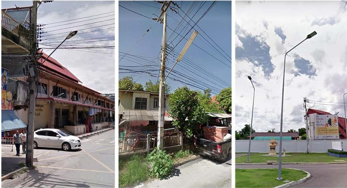
Figure 23 : Street and Outdoor Lighting in Lampang Municipality
