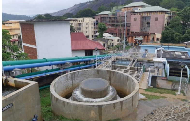
Figure 4-3) Water Treatment Plant (2)
