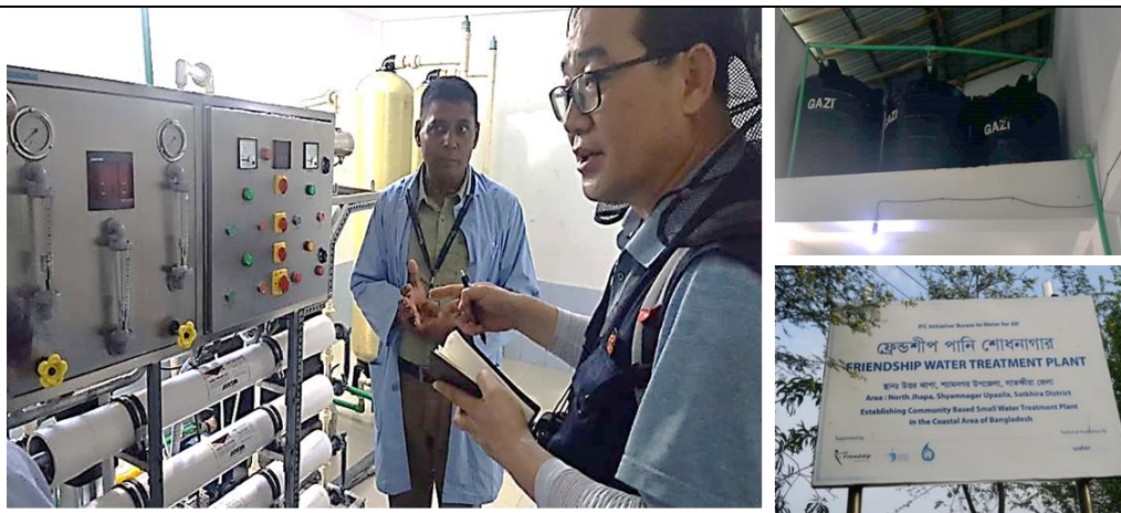
Figure 32. Reverse osmosis drinking water facilities in North Jhapa village
