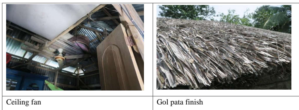
FIGURE 24 INDOOR VENTILATION AND TEMPERATURE CONTROL SYSTEM AND ROOF PROTECTION
