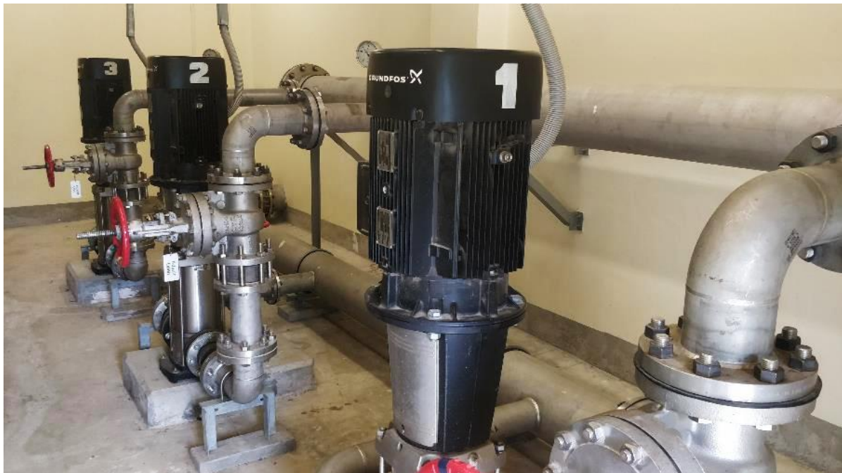
Figure 7 Borderline transfer pumps
