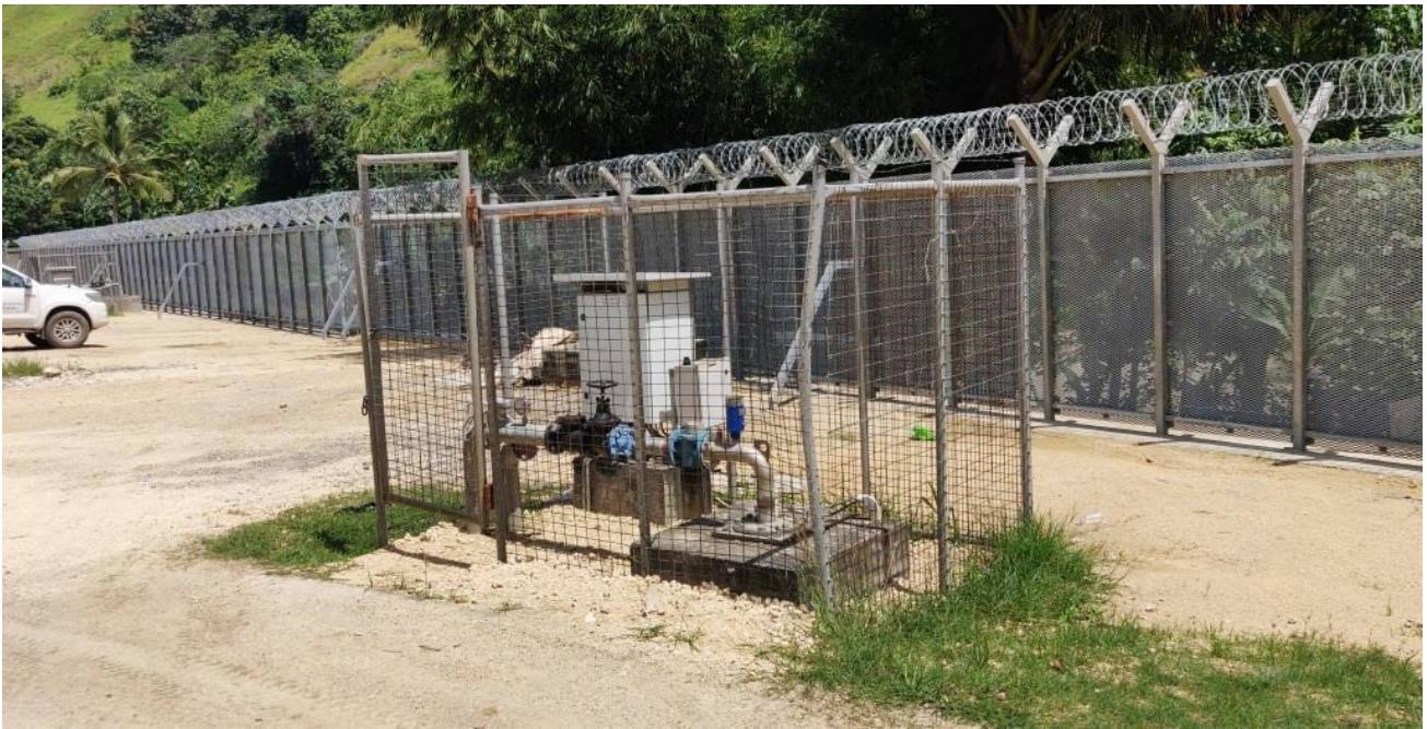
Figure 8 Typical borehole pump – Tuvaruhu
