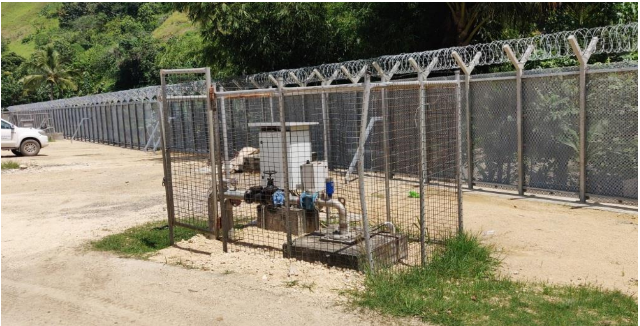
Figure 8 Typical borehole pump – Tuvaruhu
