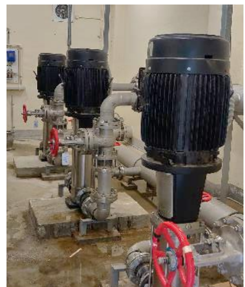
Figure 7 Titinge transfer pumps
