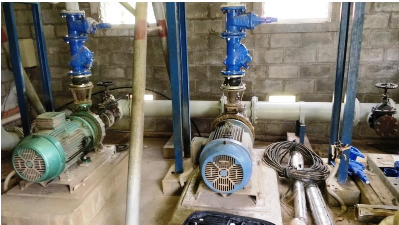
Figure 7 Tuvaruhu JICA transfer pumps
