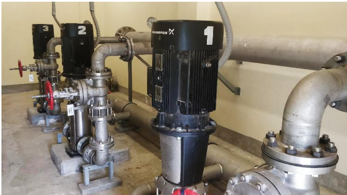
Figure 7 Skyline transfer pumps
