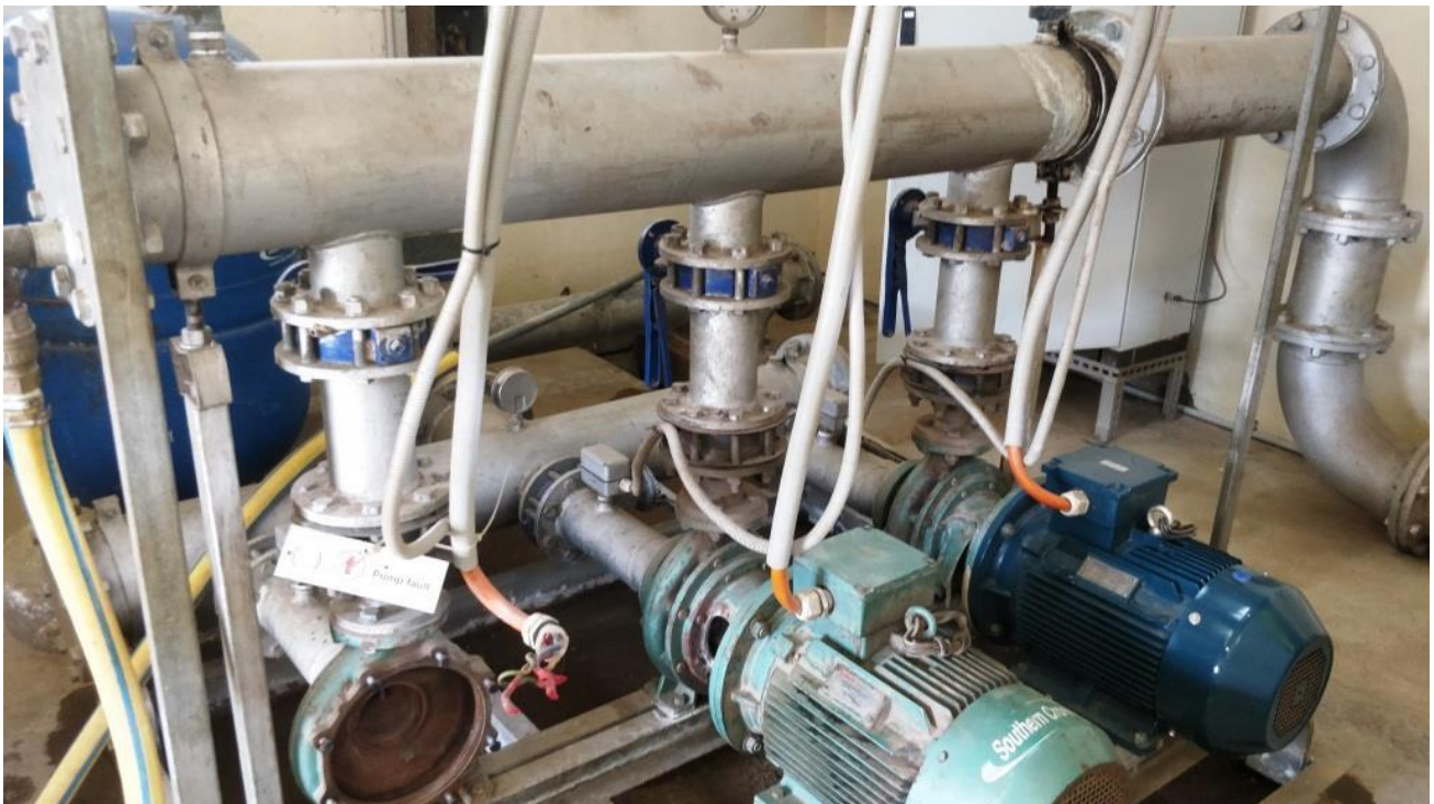
Figure 7 Tuvaruhu SIWA transfer pumps
