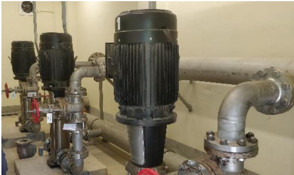
Figure 7 Tasahe transfer pumps
