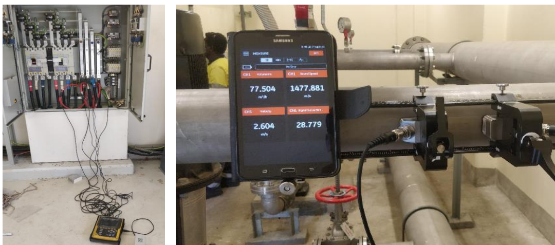
Figure 12 Power and water flow measurement photographs
