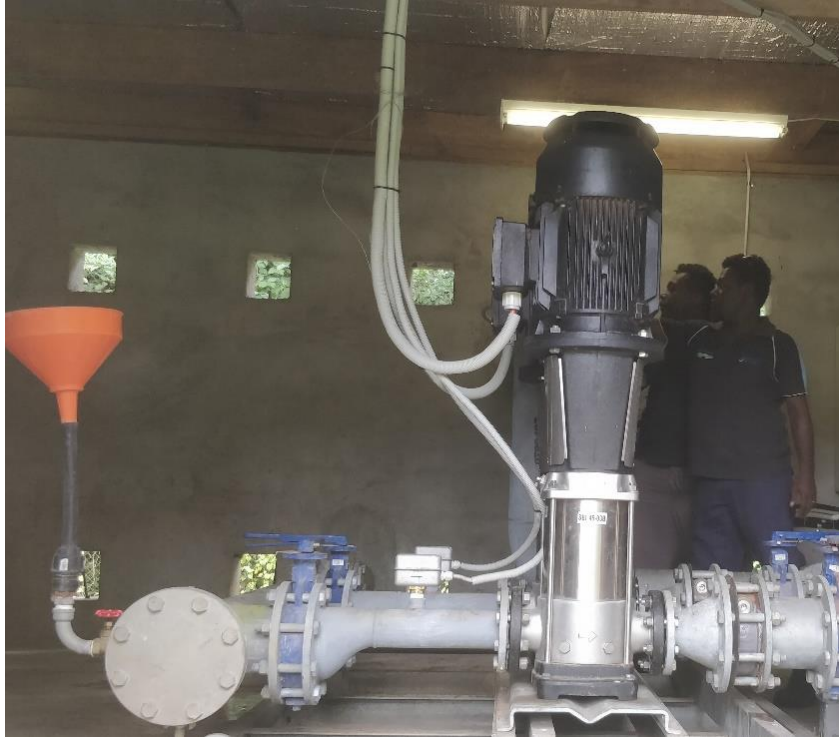
Figure 6 Kwaibala transfer pumps
