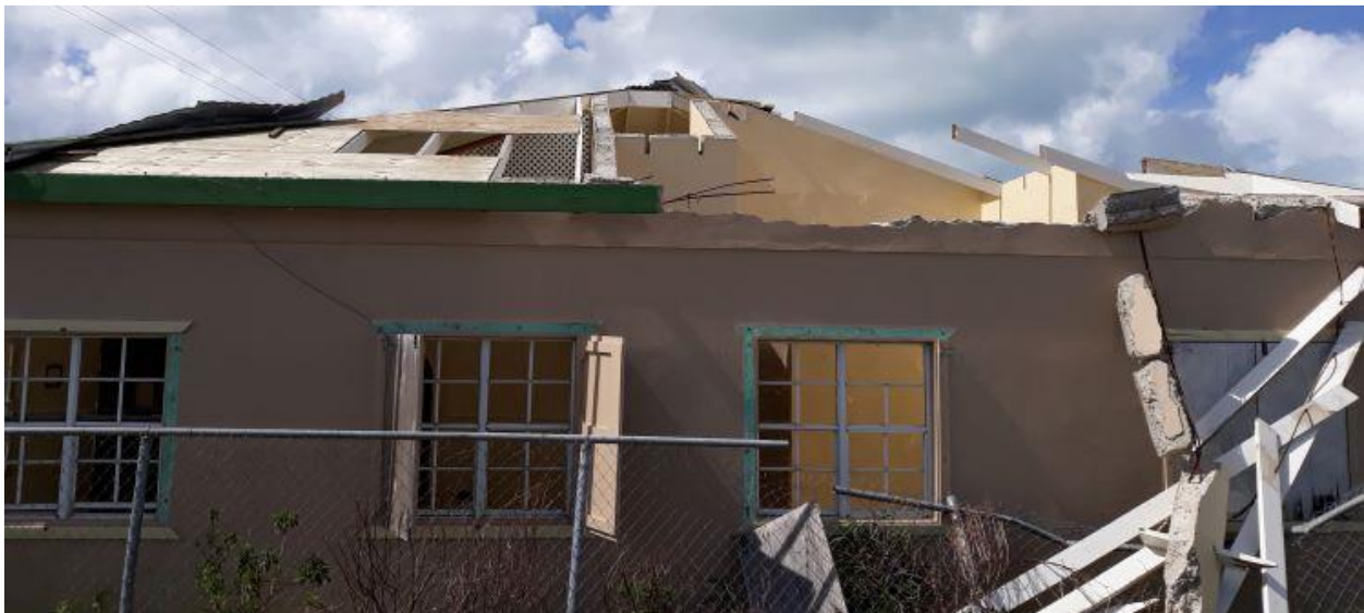
Barbuda fire station, showing multiple modes of roof failure
