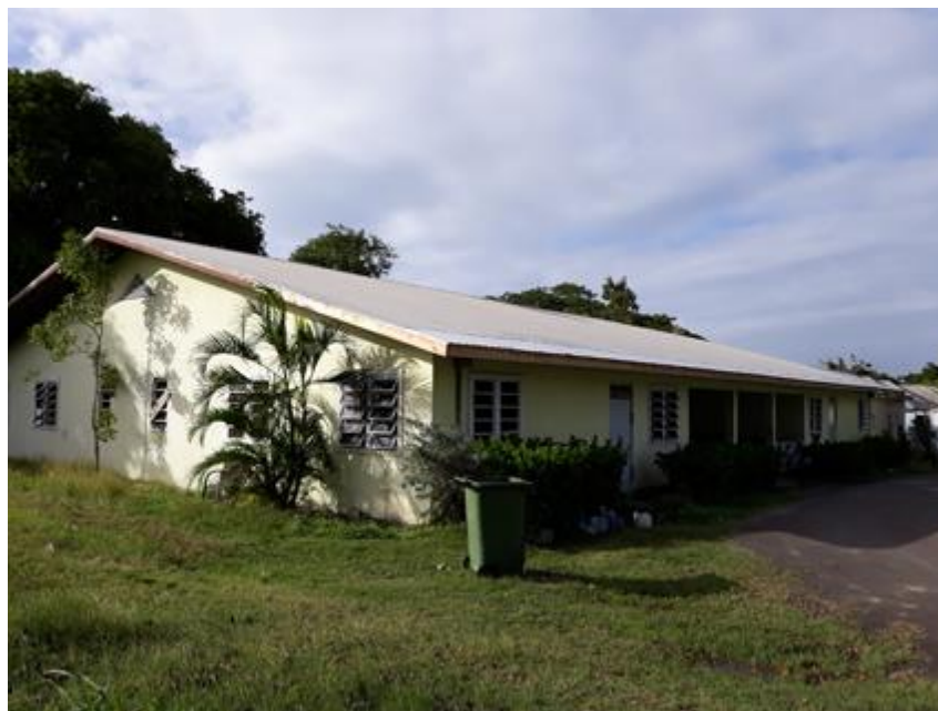
Clearvue psychiatric hospital Note the typical wood framed and sheet metal pitched roof
