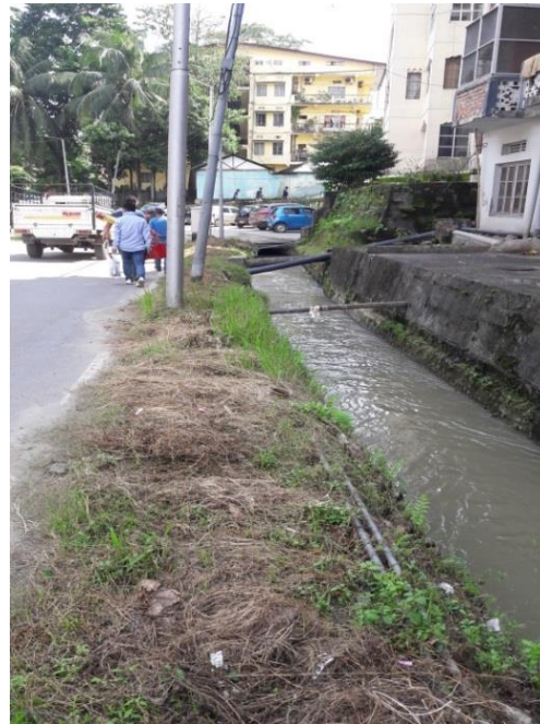
Figure 8: Irrigation canal in lower market
