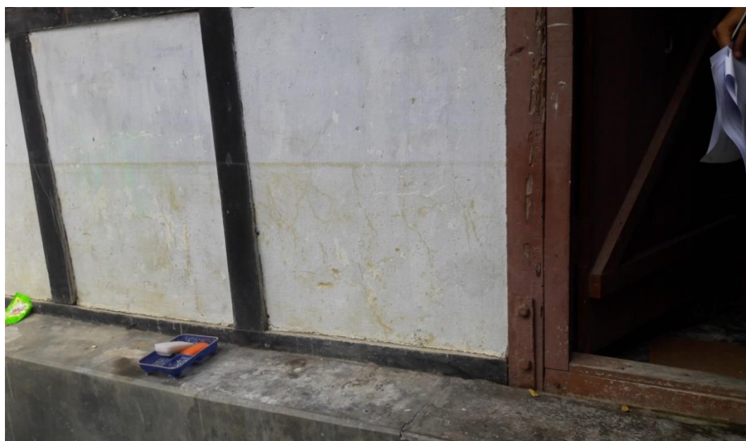
Figure 13: Flood mark on temporary structures from the 2015 flooding event
