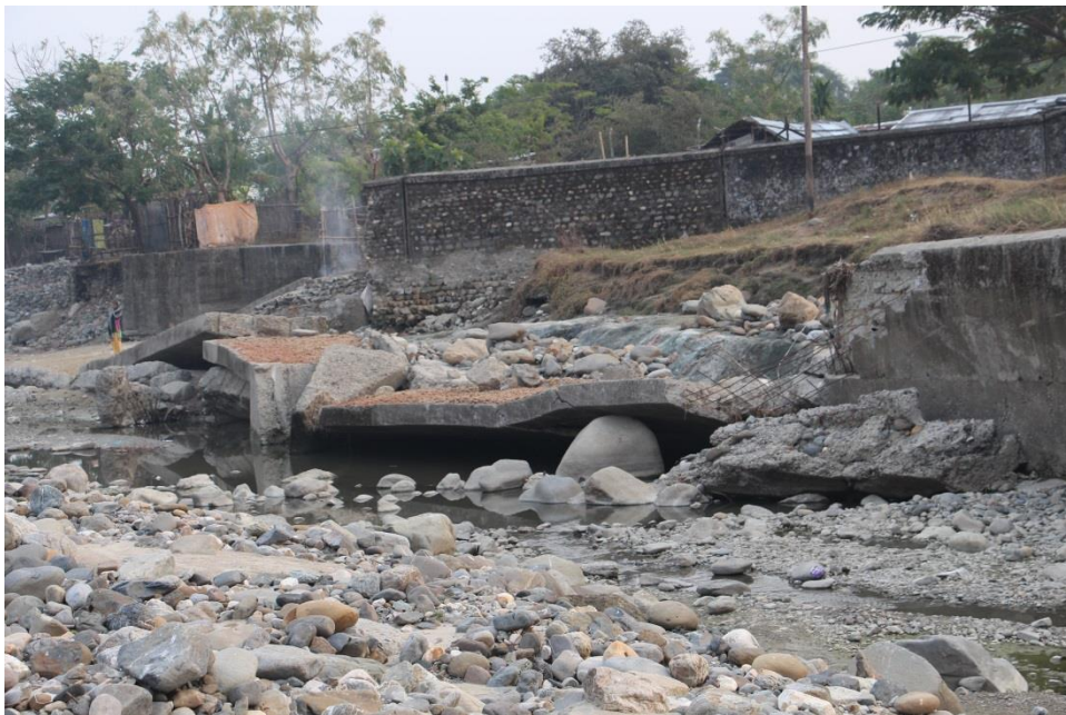
Figure 7: Damaged wall near international border
