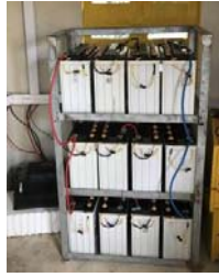
Lead-acid Battery Bank
