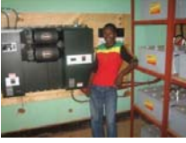
Lead-acid Battery Bank
