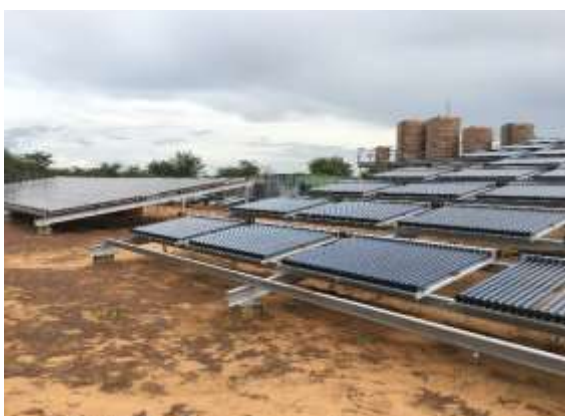
Figure 6 Akutsima Desalination Plant - Namibia
