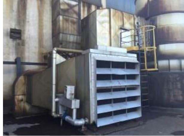
Figure 16: Hot Water Air Heater
