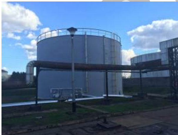
Figure 21: Aboveground HFO Tank with 10,000 m 3 Volume, Thermally Insulated
