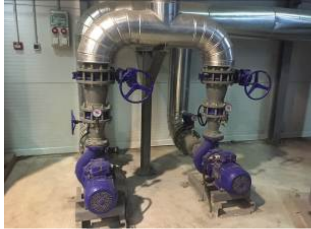
Figure 20: Main Circulation Pumps
