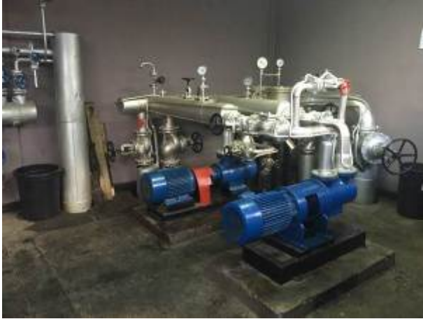
Figure 23: Circulation Pumps in Substation for HFO Tanks Heating
