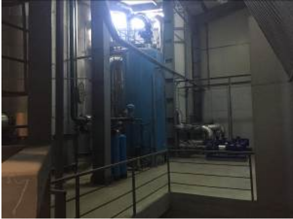
Figure 19: Platform with Expansion Modules and Circulation Pumps
