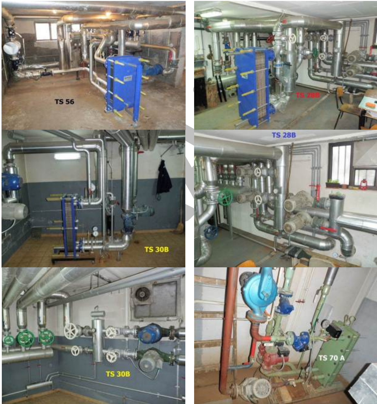
Figure 42: Installations in Substations
