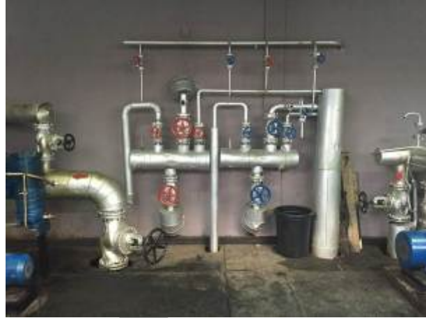
Figure 24: Splitter and Collector Located Beside HFO Tanks in Substation
