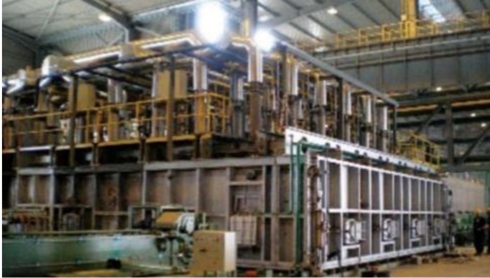
Figure 5.5: The top and-bottom firing system in use in a steel re-rolling mill
