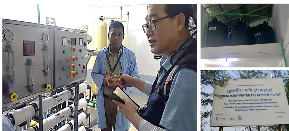
Figure 2-4 RO water supply system in village of North Jhapa
