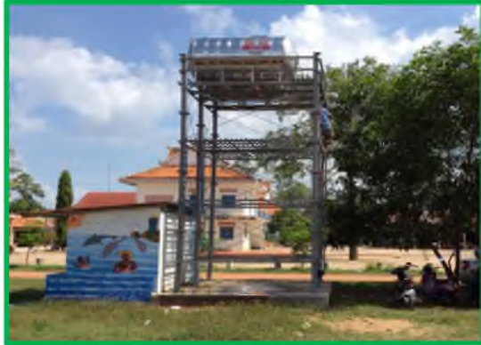
Mokmbul Primary School(Cambodia) Drinking Water 20m 3 /d (Jan. 2017)
