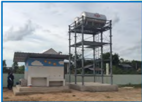
New Hope School(Cambodia) Drinking Water 20m 3 /d (Jul. 2017)
