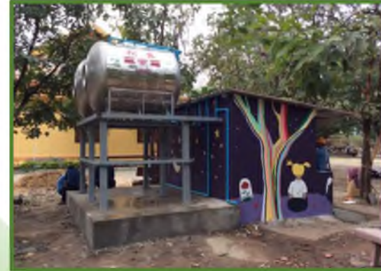
Tirumkaet Primary School(Cambodia) Drinking Water 20m 3 /d (Dec. 2016)
