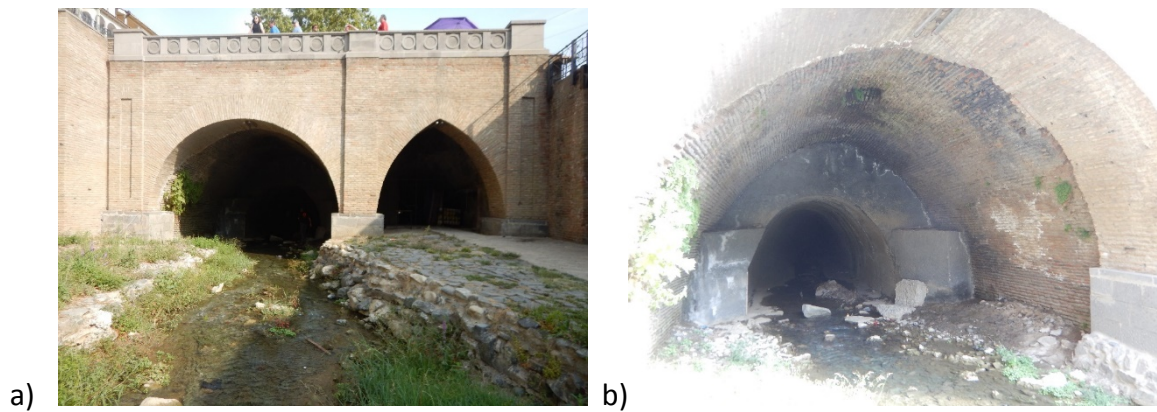
Figure 4 – Structure 1. a) Both upstream culverts, the left one opened and the right one is closed. b) Reduction in size in the left culvert
