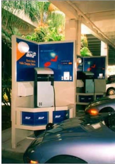
Figure 5-11. Level 2 public charge station in a mall parking structure with lighting, access control system, and a customer service speaker phone
