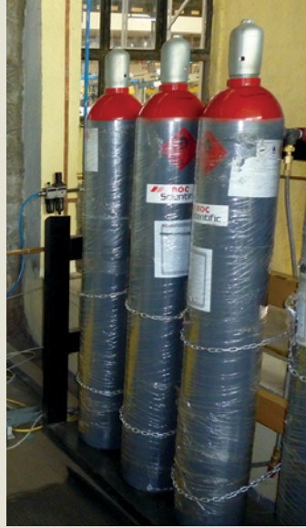
Figure 10.3 Storage of Refrigerant Cylinders
